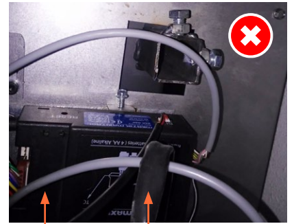
LED module cable Ignition cable
